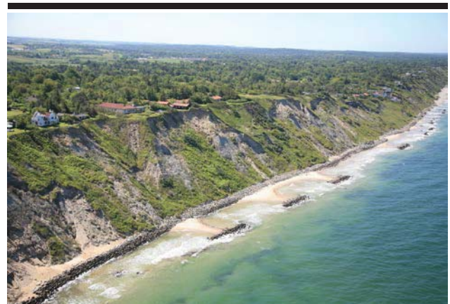
Figure 2. NE Sealand coastline with older as well as new houses on the cliff top (Photo: DCA/Hunderup Aerial Photo).
