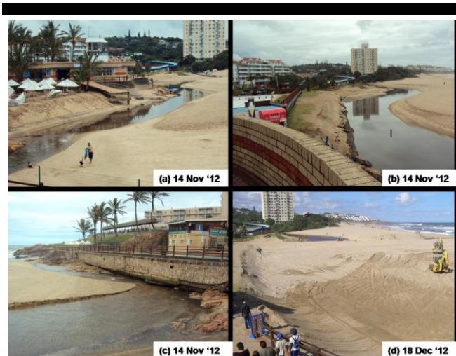
Figure 4. Margate beach (a) erosion of the ramp in front of the lifeguard tower and reduced back-beach area, (b) erosion of the embankment in front of the Olympic-size swimming pool, (c) undermining of infrastructure supporting a smaller swimming pool at the extreme southern end of Margate beach, and (d) a similar view to (b) showing infilling of the back-beach area and draining of the previously southward extending outlet; the newly excavated channel and berm to prevent southward movement of the outlet can be seen in the distance.
