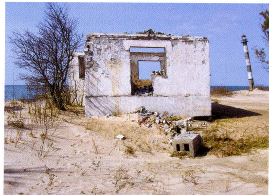
■ Figure 4.7 The former lighthouse keeper house has been destroyed by various factors, including Soviet army destruction and purely natural processes. Eventually, it will be completely destroyed by coastal erosion
