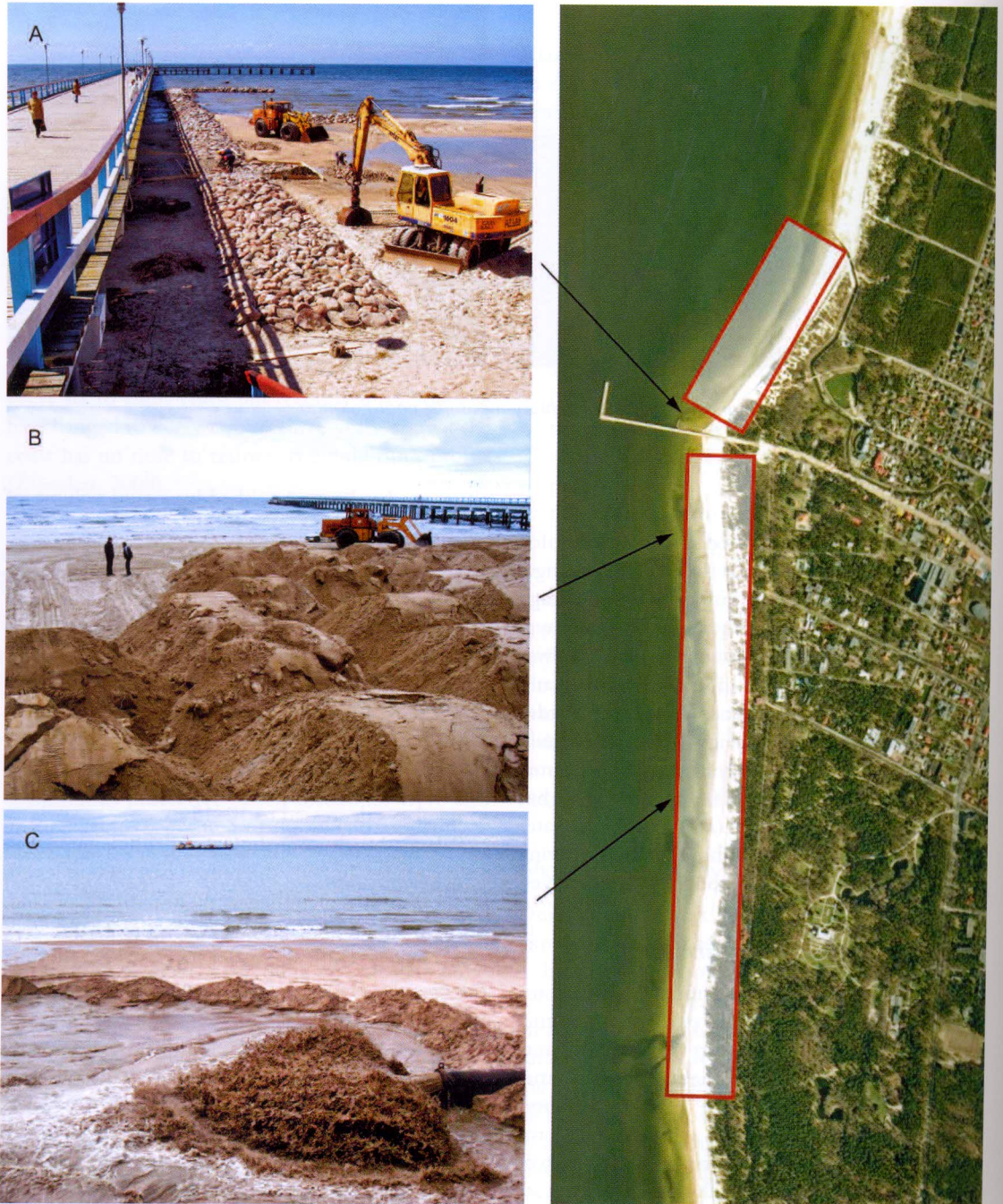
■ Figure 4.29 Palanga beach regeneration area (right): building of groin (a); beach nourishment (b, c)
